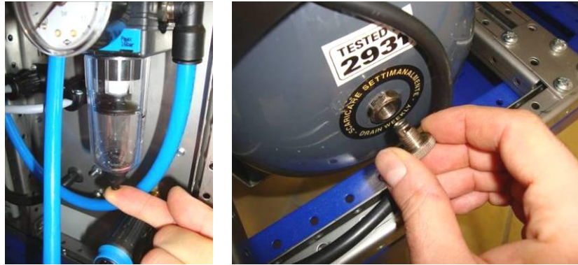
Figure 39: Draining condensate from pneumatics
